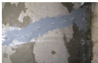
Wet Surface Crack
