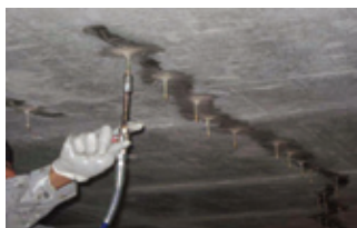
Dry Surface Crack
